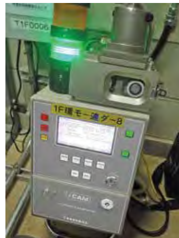
Photo by courtesy of TEPCO
